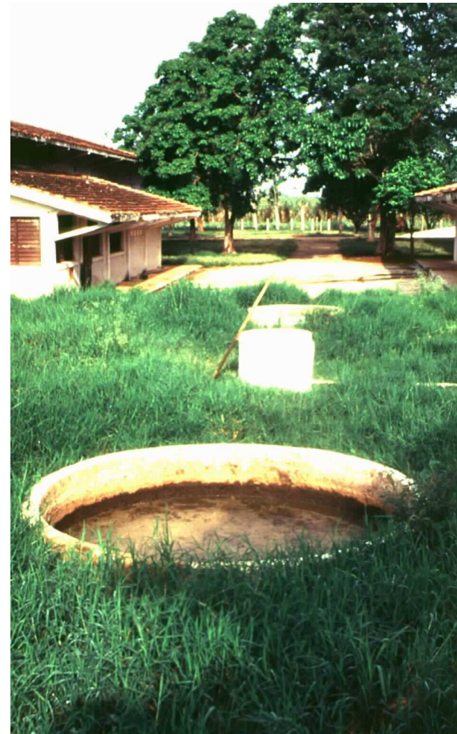
Right: Overflow (front), gas collector and off-take pipe (centre), feeder funnel (back) of a biogas fermentation chamber
